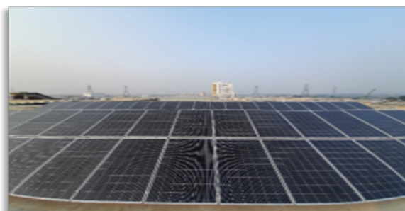
Installation of solar rooftop of the RFL building at Habiganj Industrial Park (HIP). Photo: courtesy
