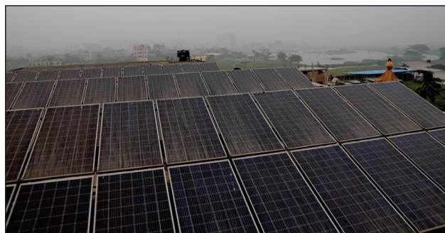
Rooftop solar PVs.
